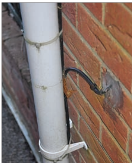
Fig. 6a: Feeder partially concealed behind a plastic downpipe. The black feeder used here illustrates the idea.
